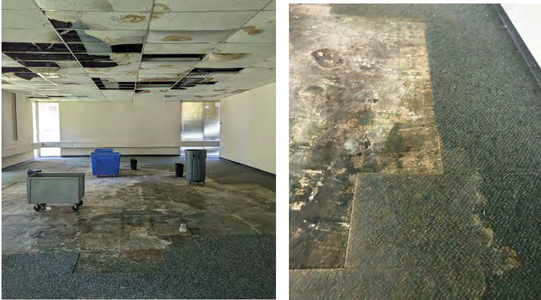
Figure 12 (Left)– Extensive corrosion within floor and ceiling tiles. Figure 13 (Right) – A deteriorating rug, lined with mold.
