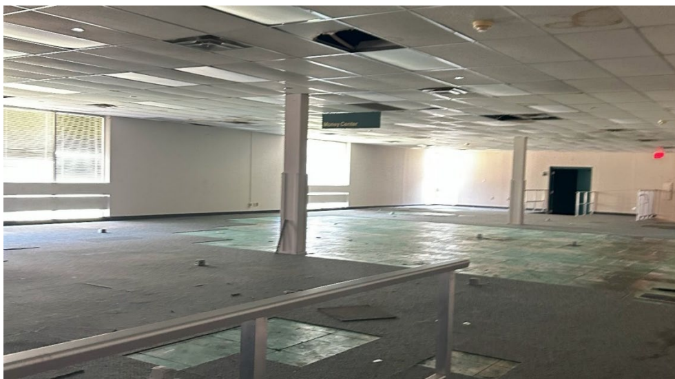
Figure 11 – Overview of the former Money Center, now entirely vacant and deteriorated.
