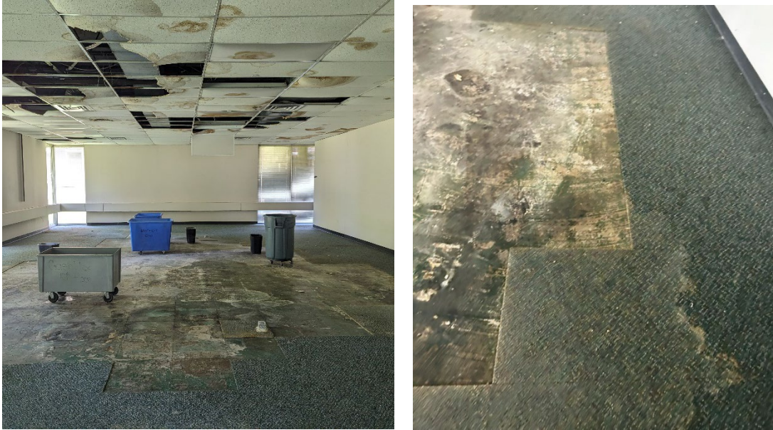
Figure 12 (Left)– Extensive corrosion within floor and ceiling tiles. Figure 13 (Right) – A deteriorating rug, lined with mold.
