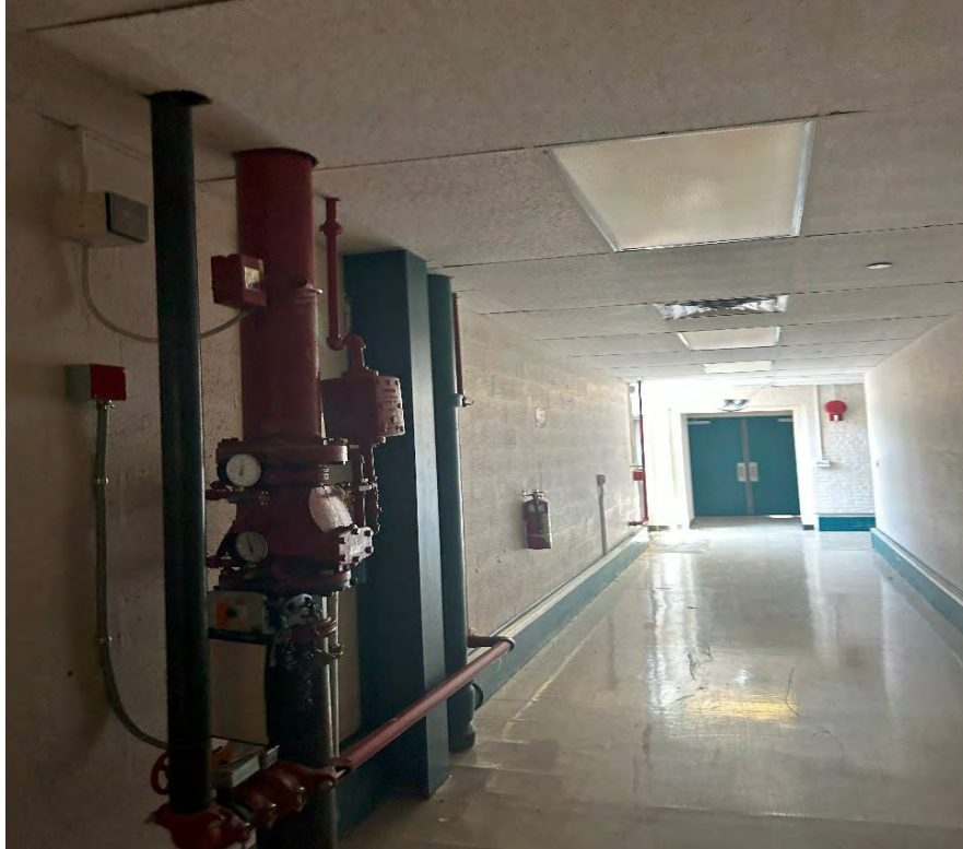
Figure 21 – Exposed piping and meters within the hallway of Building 180.
