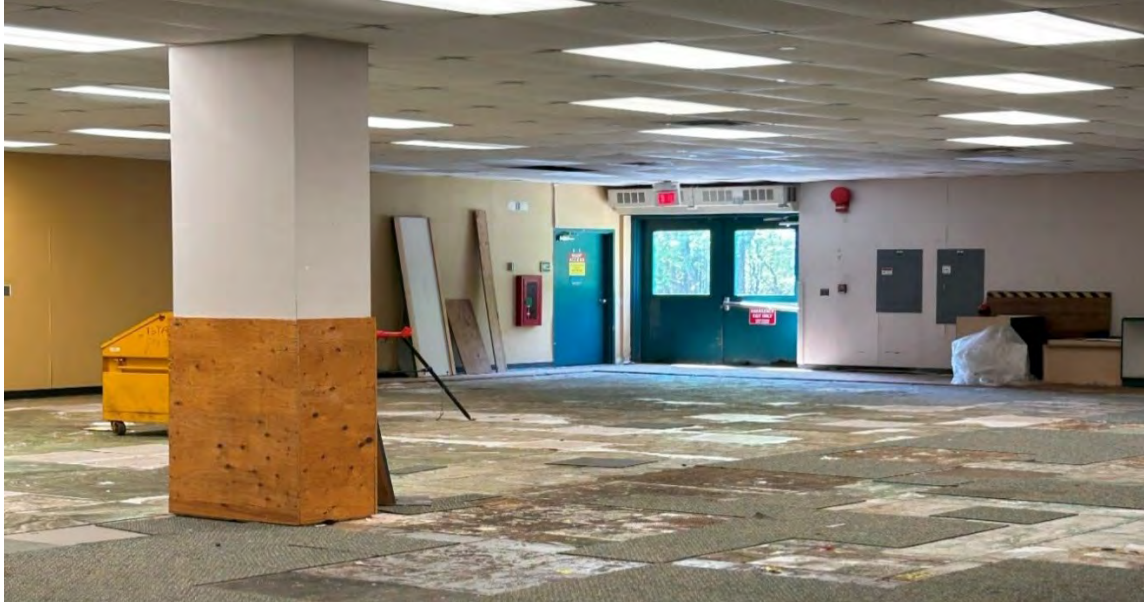
Figure 18 – Damaged floor tiles and wrapped column within the old Data Center.
