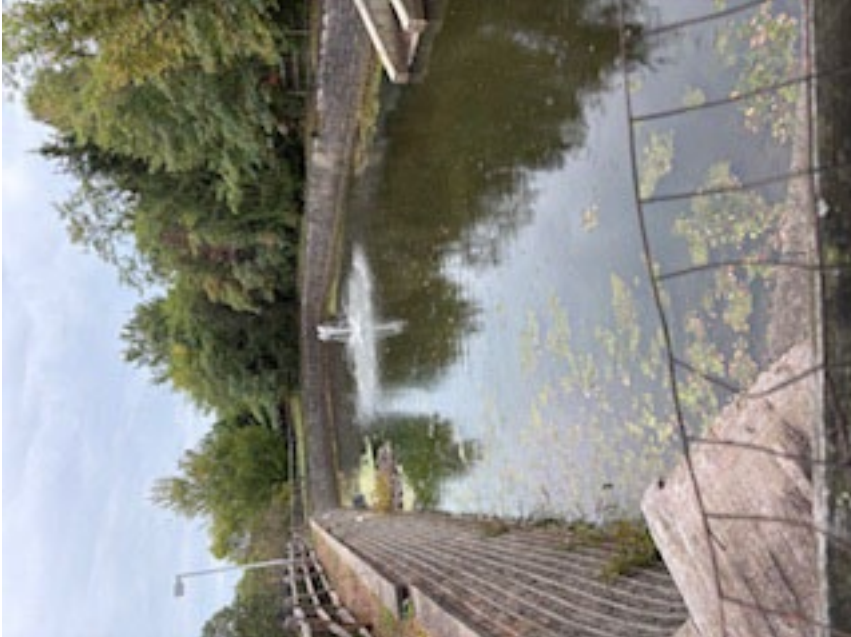
Bad retention pond example
